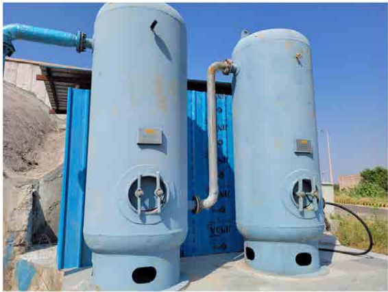
High-Pressure Storage Facility
